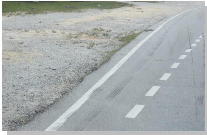
Rajah 9 : Unpaved Gravel Shoulder
